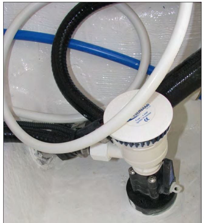
Port Release Well Pump & Seacock ON/OFF Valve
