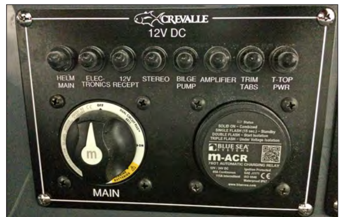
Battery Switch Panel Battery Selector Switch and Circuit Breakers
