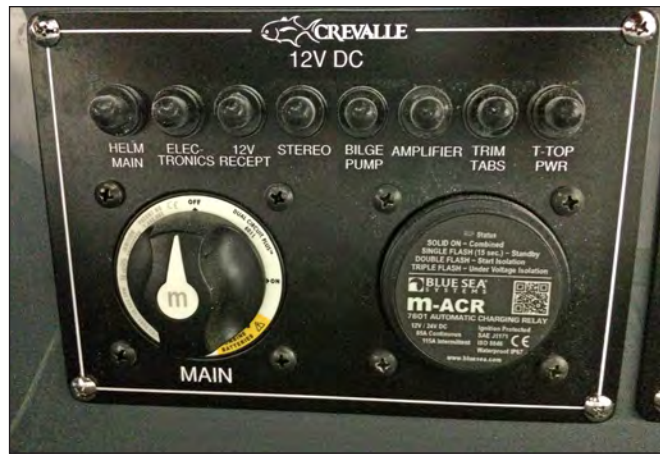
Battery Switch Panel Battery Selector Switch, ACR & Circuit Breakers
