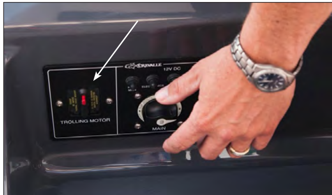
Typical Trolling Motor Circuit Breaker
