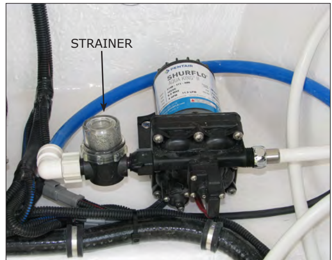
Fresh Water Pump and Strainer
