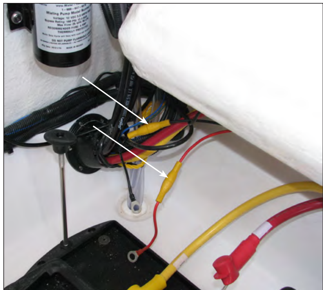
Battery Charger Output Wire Circuit Protection
