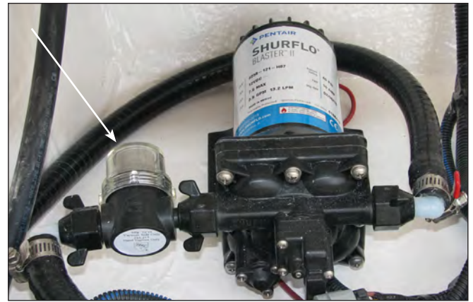
Raw Water Pump Strainer
