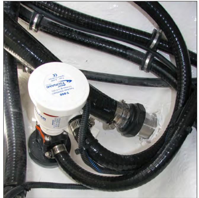
Starboard Release Well/Baitwell Pump & Washdown Pump Supply Hose Fitting
