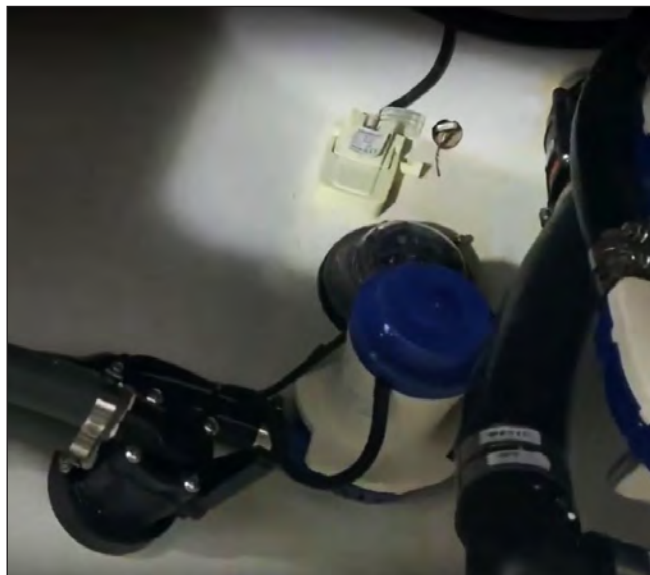
Aft Bilge Pump & Automatic Switch
