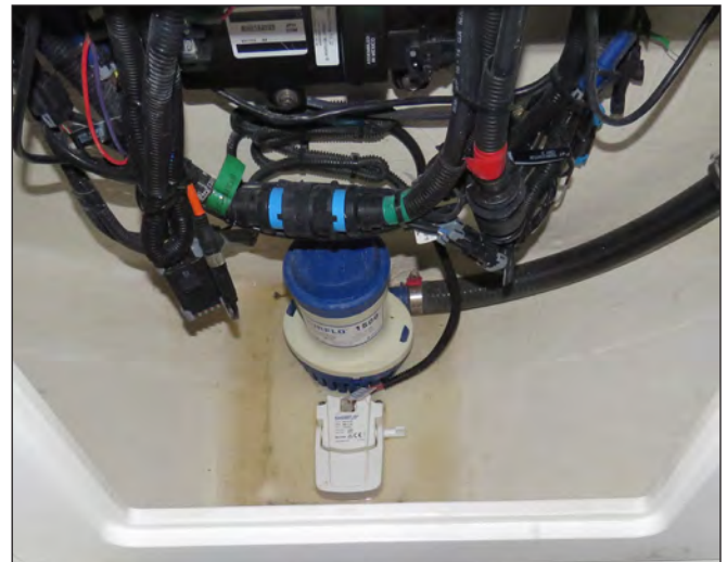
Forward Bilge Pump & Automatic Switch
