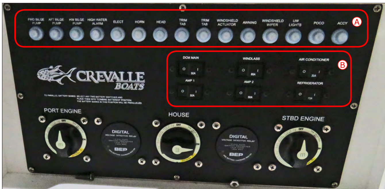
Accessory & Main Circuit Breakers In Battery Switch Panel
