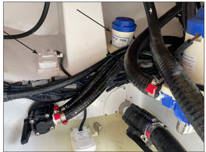
Emergency Bilge Pump & Emergency Pump & Alarm Automatic Switch
