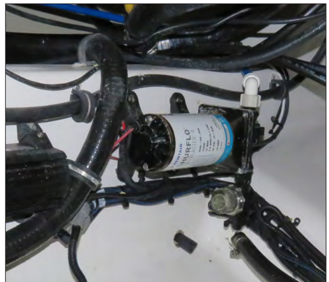
Raw Water Pump & Strainer
