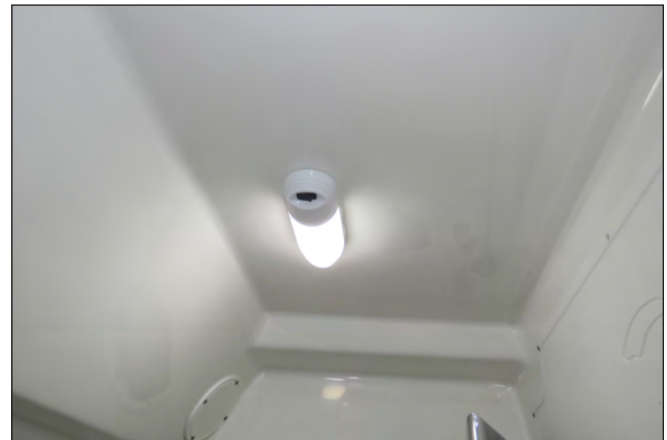
Overhead Light & Switch
