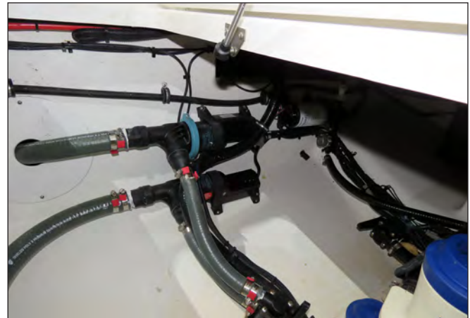
Aft Fishbox Pumps
