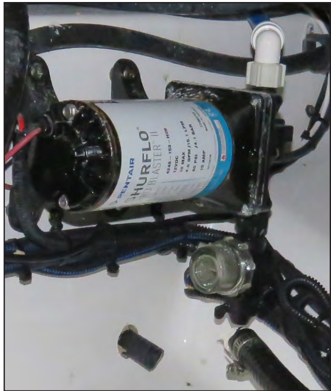
Raw Water Pressure Pump & Sea Strainer
