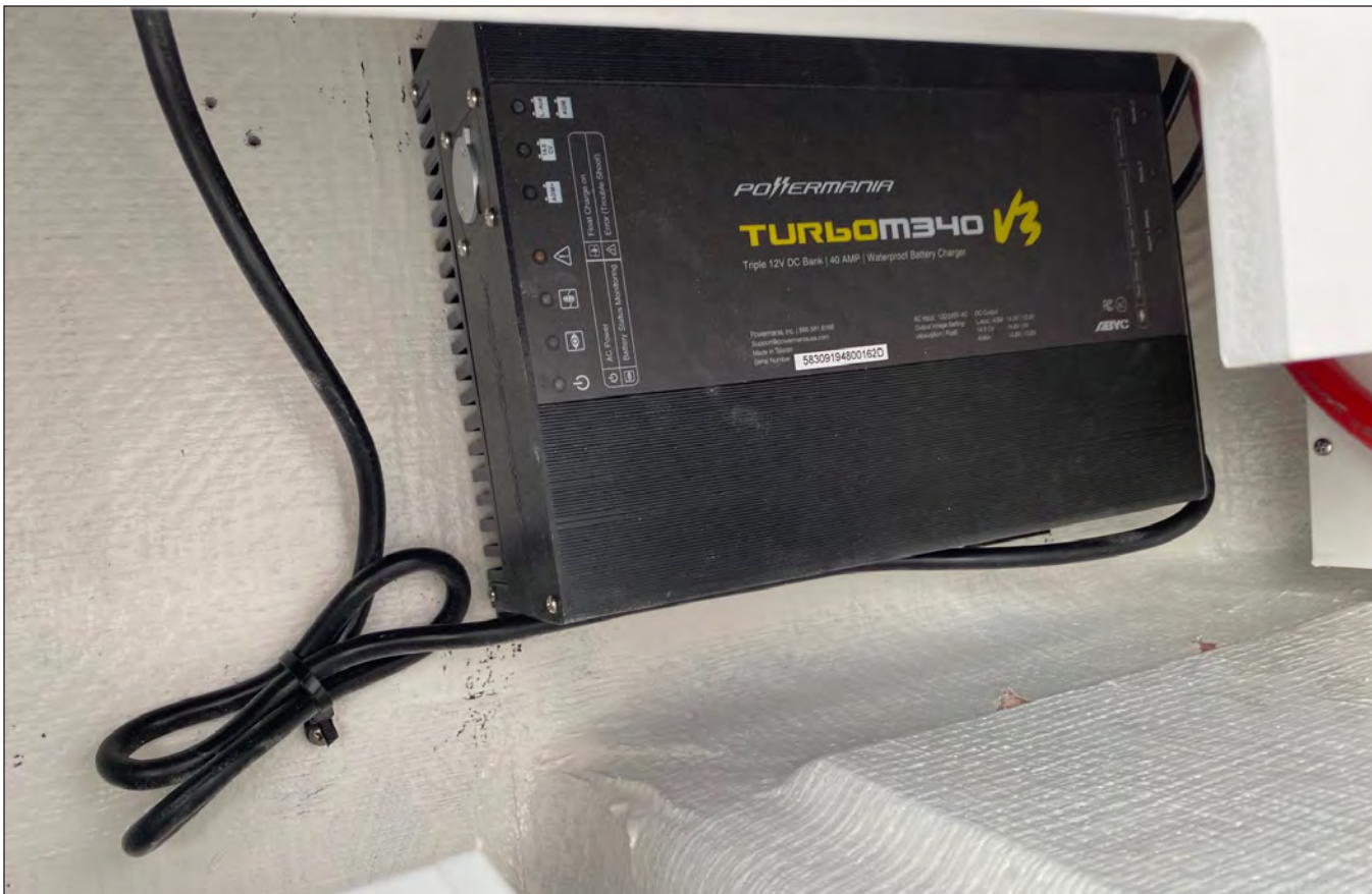
Typical Battery Charger
