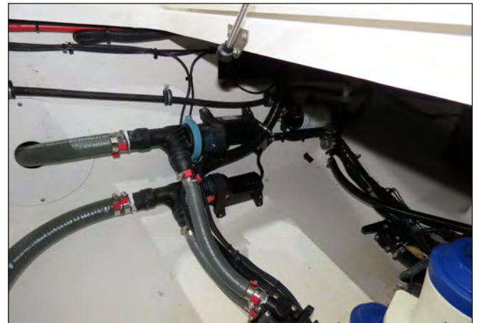
Below Deck Fishbox Pumps
