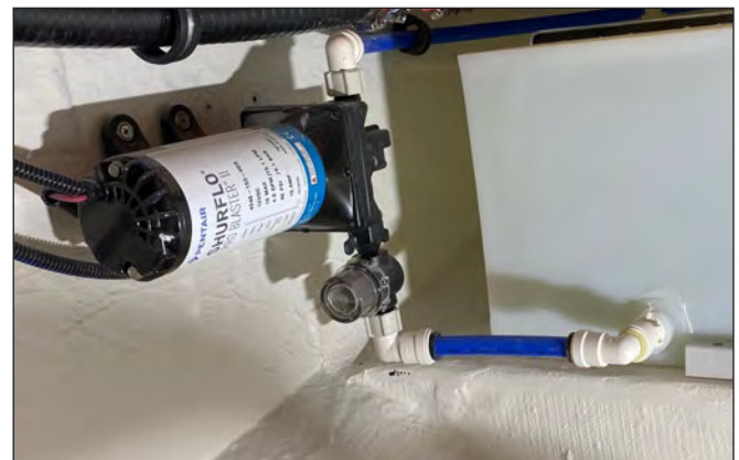
Fresh Water Pump & Strainer
