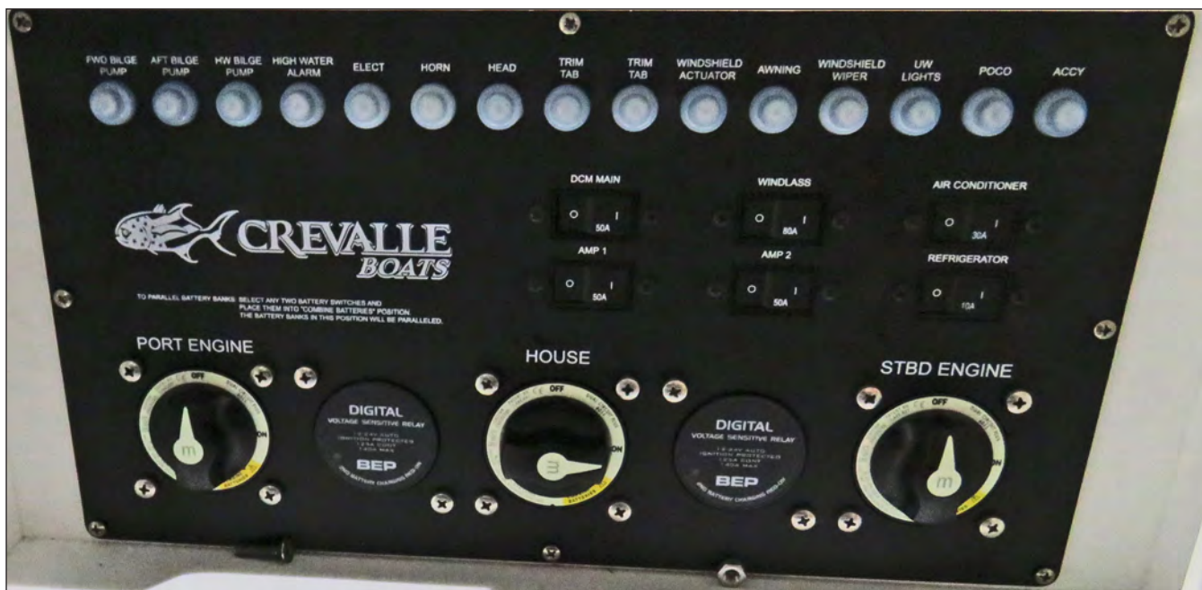
Battery Switch Panel, Battery Switches, Main Circuit Breakers & Accessory Breakers
