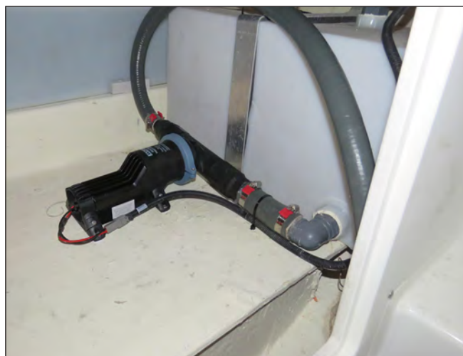
Waste Overboard Discharge Pump & Holding Tank
