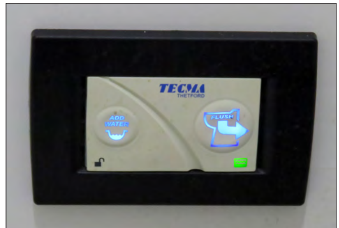
Head Control Panel
