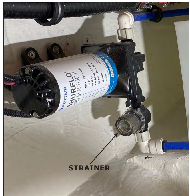
Typical Fresh Water Pump & Strainer
